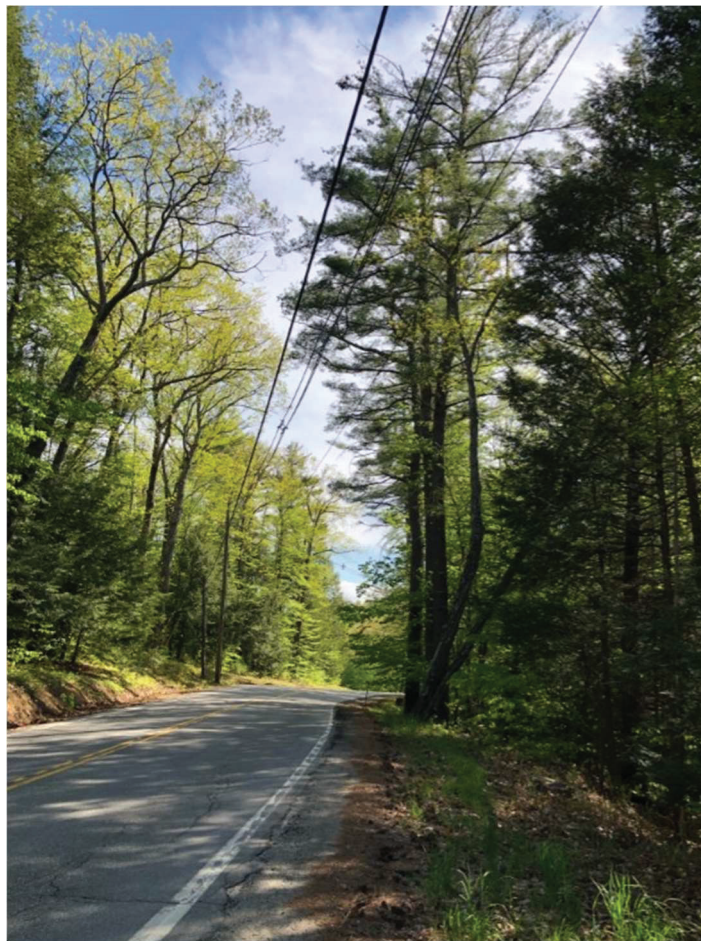
Figure 5-51. Eversource Line Reconductored to Spacer Cable
