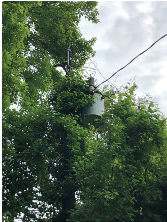
Figure 5-24. Vegetation on Distribution Transformer Pole
