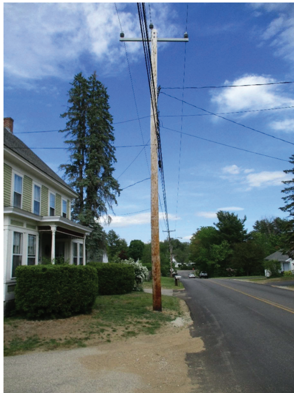
Figure 5-6. Example of Class 2 wood pole with fiberglass crossarm
