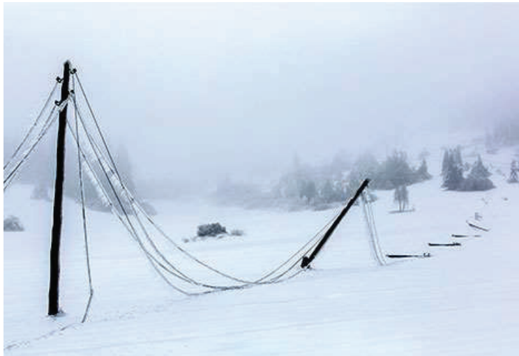
Figure 5-2. Illustrative example of wood pole failure due to ice loading
